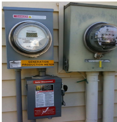
Figure 44- Generation Production Meter and Disconnect Switch Location
