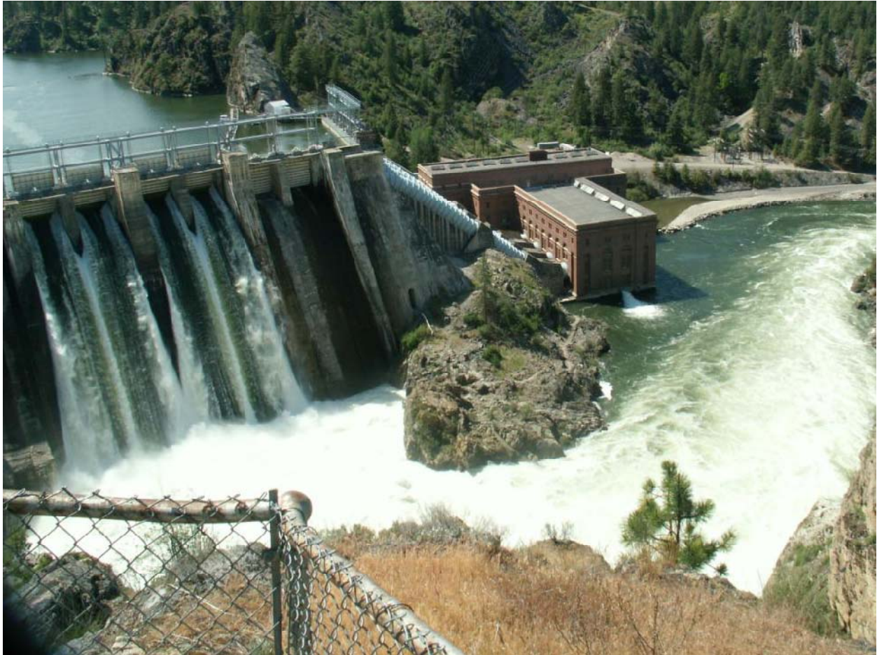
Plate LL1. Long Lake Dam and Powerhouse as Viewed From Overlook, May 22, 2008 at 09:45 PDT
