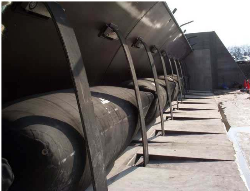
Plate NM2. Example of Pneumatic Controlled Spillway Control Structure Manufactured by Obermeyer Hydro Inc.
