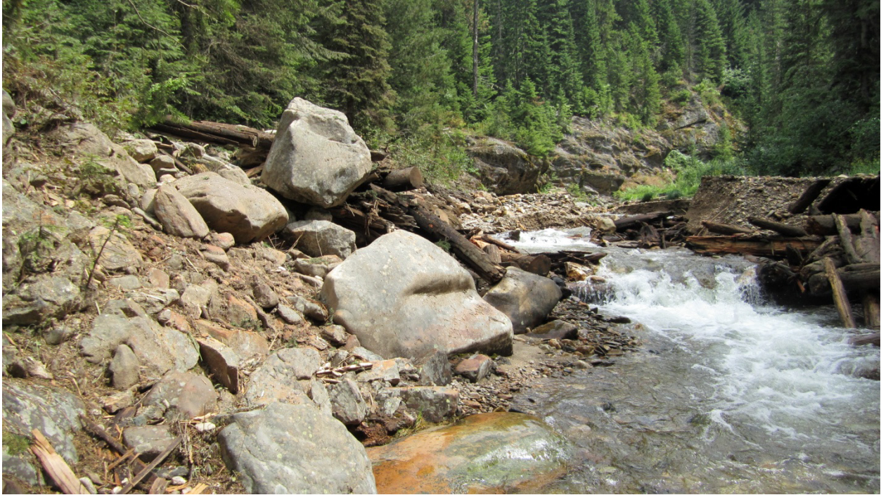
Figure 5. Upper Marble Creek Splash Dam after the Passage Breach, Summer 2014.
