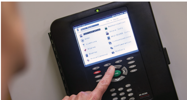
Rosauers uses an automated energy management system to fine tune everything from lighting to refrigeration temps.
