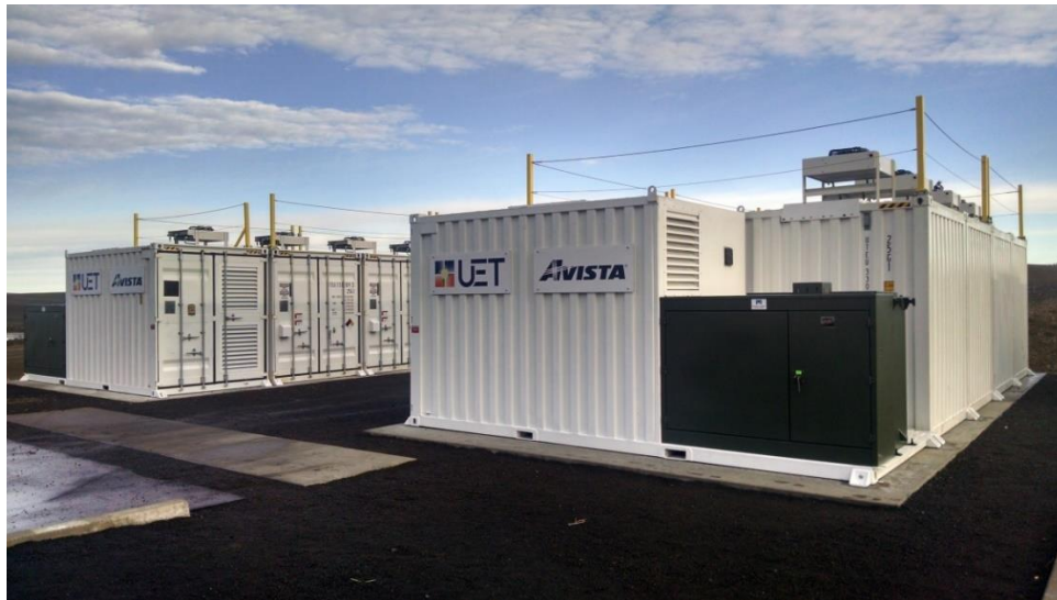
Turner Energy Storage Project, Pullman, WA
