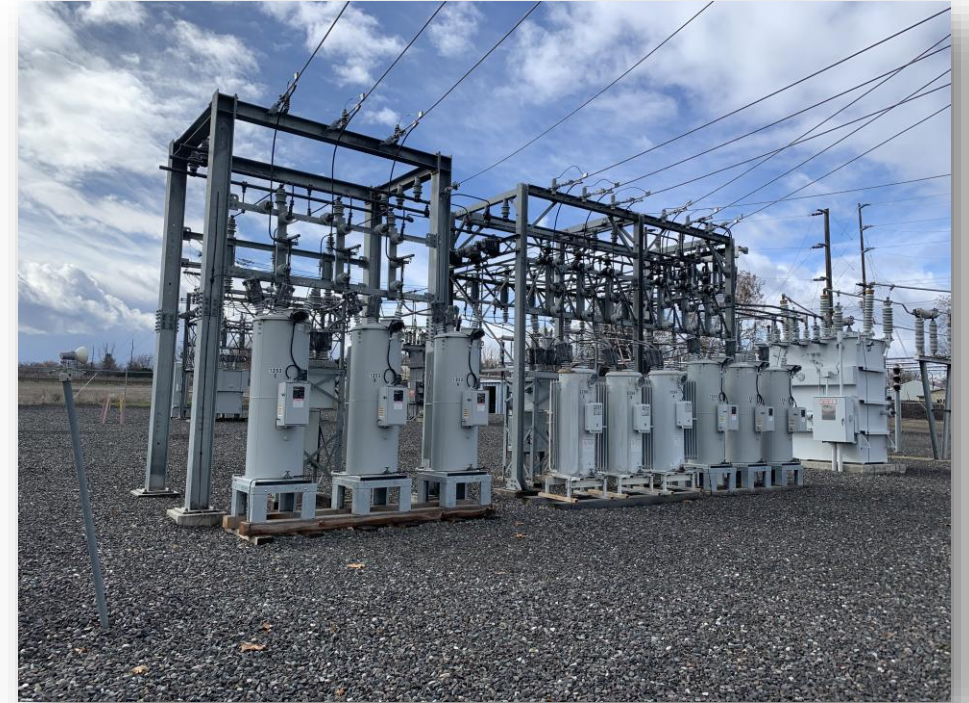
Avista's Tenth & Stewart 115kV / 13kV Substation, Lewiston, ID
