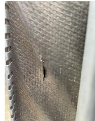
Tear in Fabric Duct Transition
