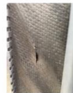
Tear in Fabric Duct Transition
